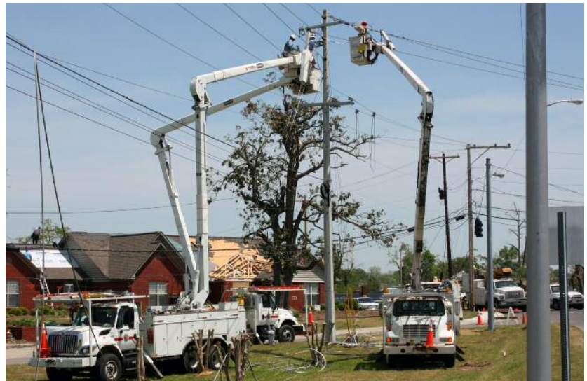
In April of 2010 Huntsville Utilities crews went to Albertville, AL to help restore service after an EF3 tornado ripped through the town on April 24th.
