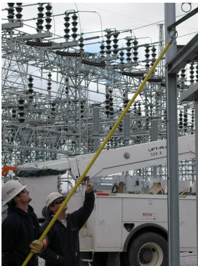
Electricians prepare to close a circuit in a large substation in downtown Huntsville. Huntsville Utilities had 93 substations serving nearly 164,000 customers in an area of over 800 square miles during FY2010.
