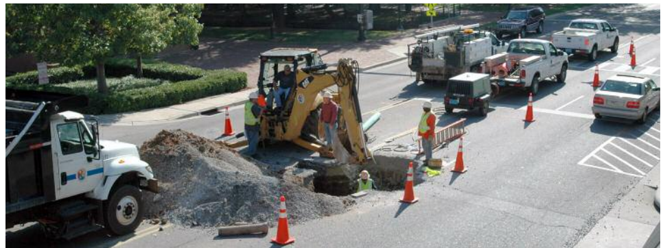
A water crew works on a leaking pipe in downtown Huntsville. Safety cones are used to warn vehicle operators about the proximity of the utility work to the lane in which they are driving as well as to try to ensure the safety of the utility workers.
